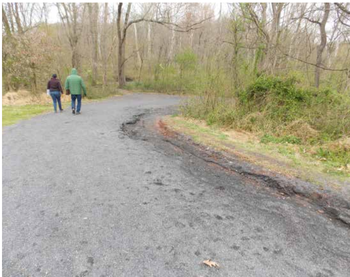
Trail along the west end of the park that often sees erosion from storm events.
