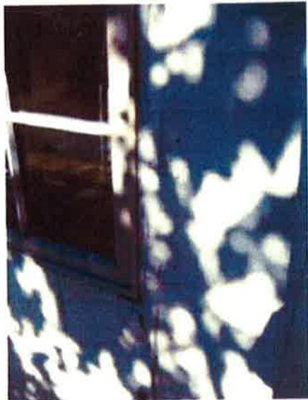
Siding at Window Rotted and Caulked Improperly
