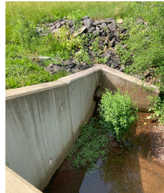
This culvert structure near the entrance drive directs an unnamed stream below Allentown Road toward the site.
