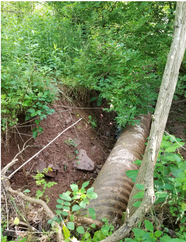
The unnamed stream exhibits signs of erosion along the culvert pipe at the low point of the site, likely from high volumes of stormwater runoff conveyed during heavy rain events.
