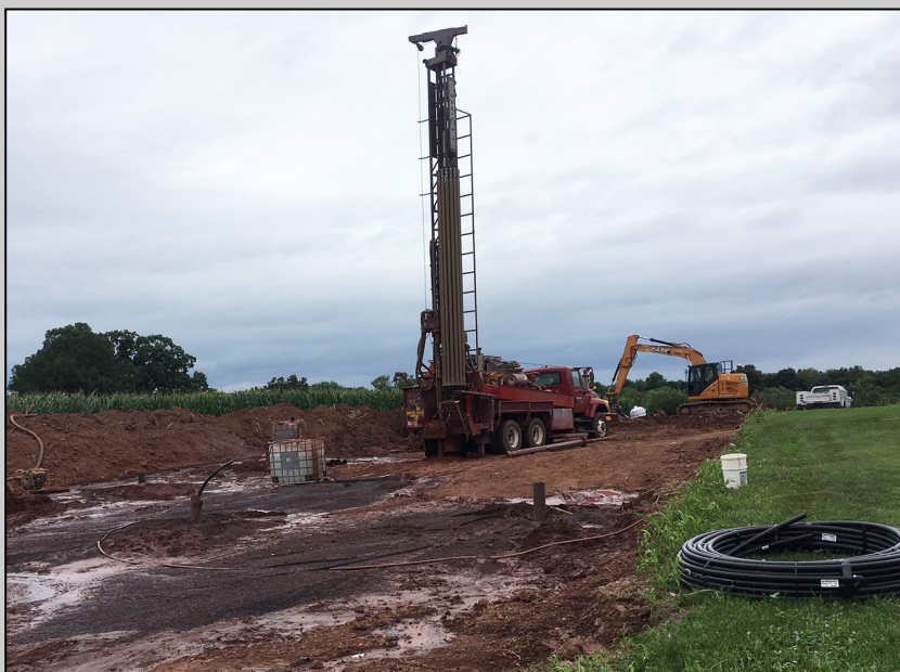
Active work zone within the well field of the future geothermal system
